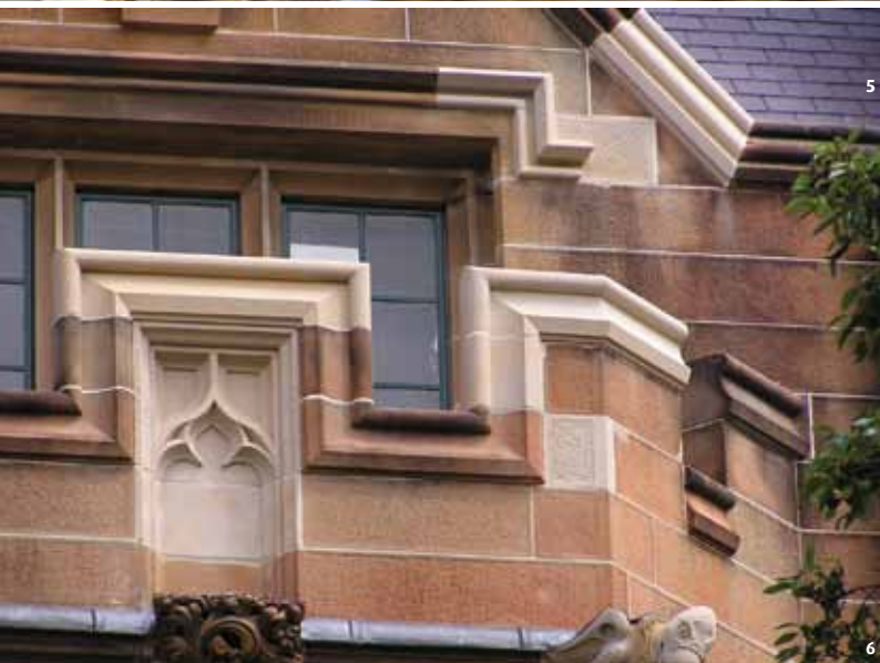
Photo 4: Replacement stone in the parapet at the State Library of NSW. Photo 5: Wholesale replacement of stone in the pediments, tower and balustrades of Sydney Observatory. Photo 6: McCaffrey's stone in the Anderson Stuart Building, University of Sydney. (Photos: Jasper Swann, 2007)
