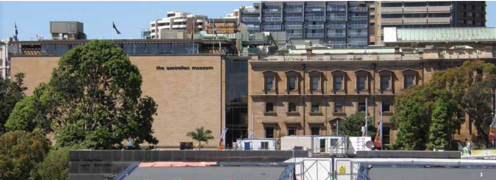
Photo 1: Art Gallery of New South Wales, restored using Capricorn Custom Buff. Photo 2: Darlinghurst Law Courts, Sydney. Photo 3: Replacement of the cornice and balustrade at the Australian Museum. (Photos: Jasper Swann, 2007)
